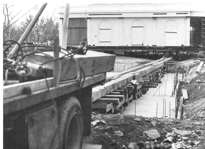
In the late 1960s, Le Petit Trianon was painstakingly moved from its original location where today's Flint Center stands to be placed on its permanent foundation at its present site. Courtesy California History Center Foundation, Stockmeir Library Archive.
