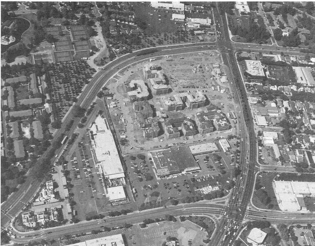
The 16-acre piece of Olson cherry orchard in Sunnyvale under construction, November 2000. Photo by 111th Aerial Photography Squadron.
